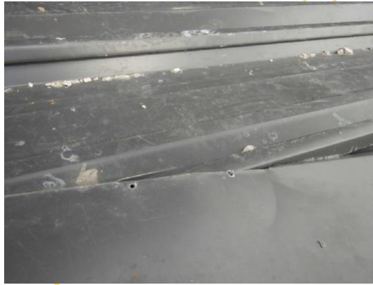
Front LHS-missing rivets
